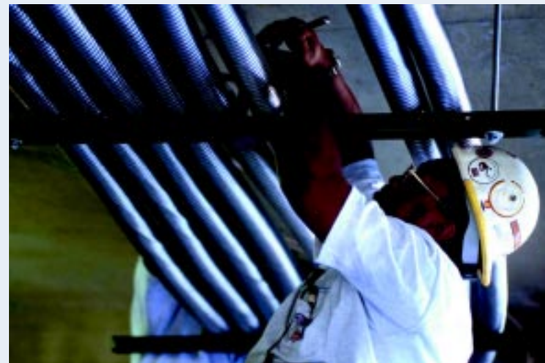
Photo 4. Horizontal supports on trapeze.
