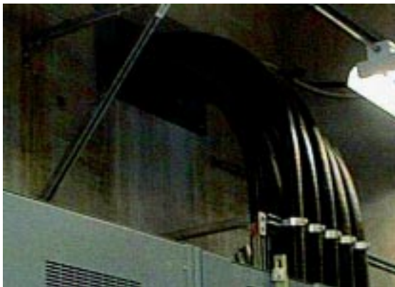
Photo 8. Parallel runs of jacketed MC cable entering gear.
